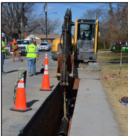
This trench along Barbee Street was quickly repaved in 2022.
