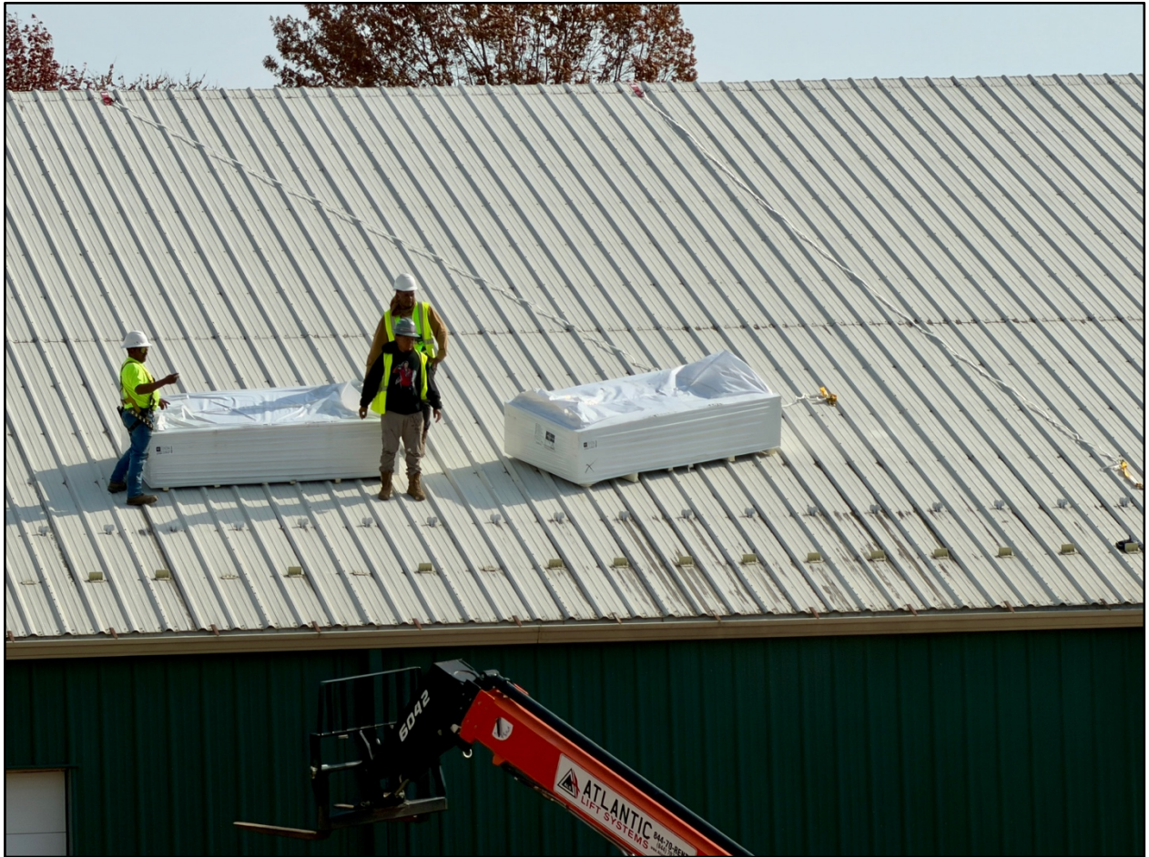
In addition to the Wellness Quarter construction, work began this week on the DWTC roof overlay.
